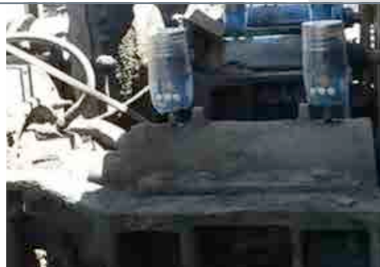
Chesterton Lubri-Cup EM applied the new, high-performance grease.
