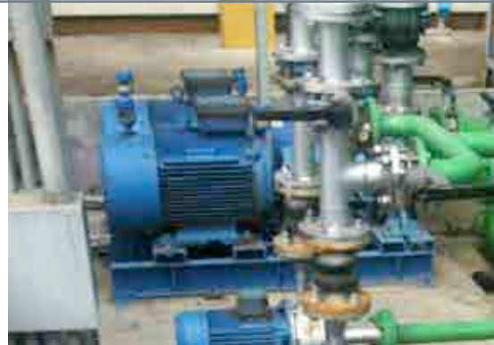
Over greasing led to frequent bearing failure.
