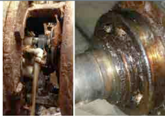
Bearing failed frequently in slurry pumps.
