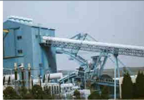
Chesterton 615 HTG #2 resists chemical attack in the coal yard.
